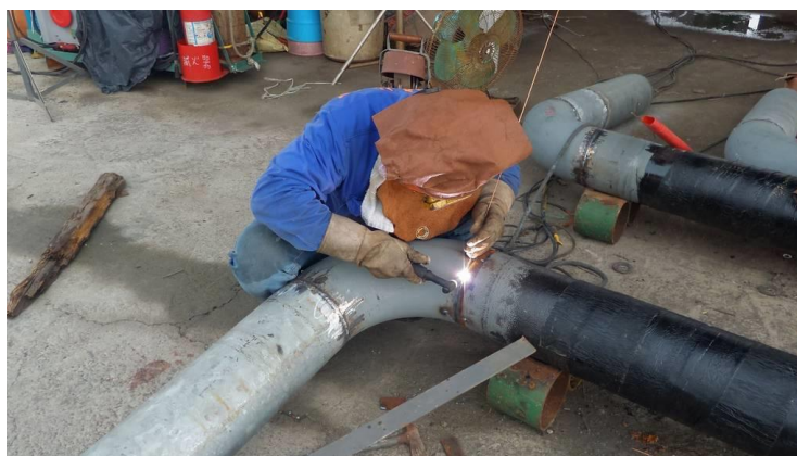
Fig. 2-5: Traditional pipe-elbow prefabrication, the ring-weld bead damage caused by high temperature
