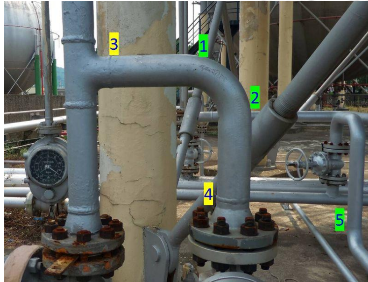
Fig. 3-2: Piping in this case - single pipebend (marked points 1/2/5 for DH Quick-Bending, 3/4 for traditional ring-weld)
