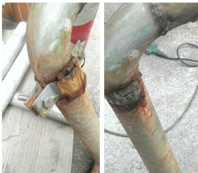
Fig. 2-6: Traditional broken pipe repair and leakage (left), and perforation leakage of the base material of the bead line (right)
