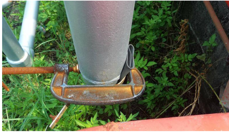
Fig. 3-1: Micro-damage of the pipeline in this case, temporary leakage (traditional ring-welding)
